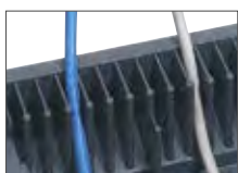
Cable held in place by guides inside the box
